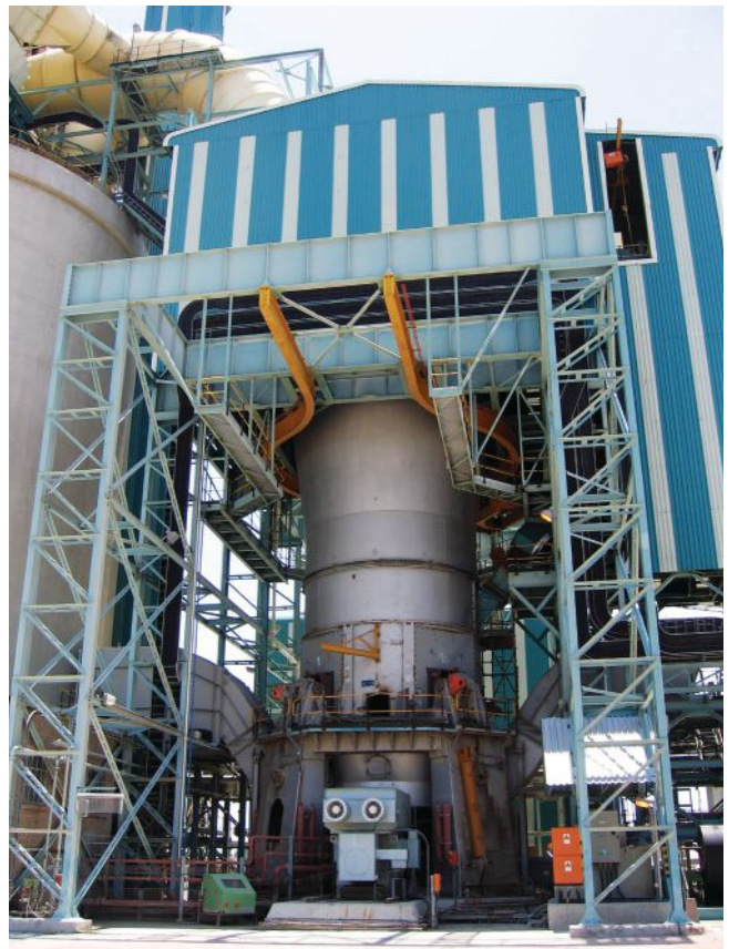
A Loesche VRM has successfully processed phosphate rock at Phalaborwa, South Africa, for 25 years.
